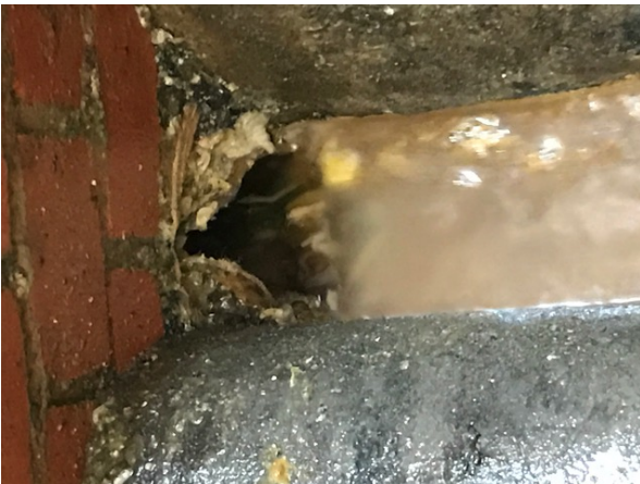
See close up of defective pipe liner in the pipe exit
