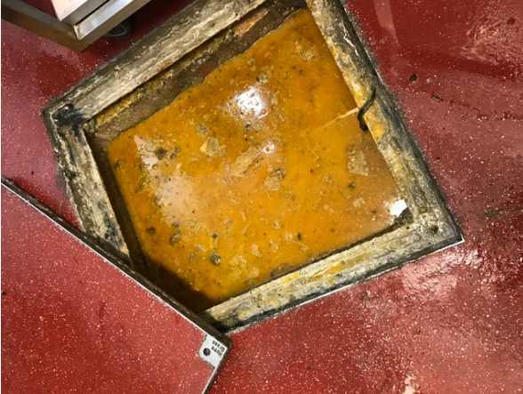
Manhole prior to emptying, see grease content
